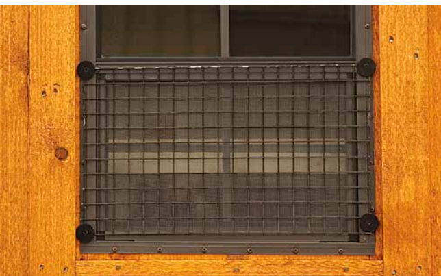
Wire over window
